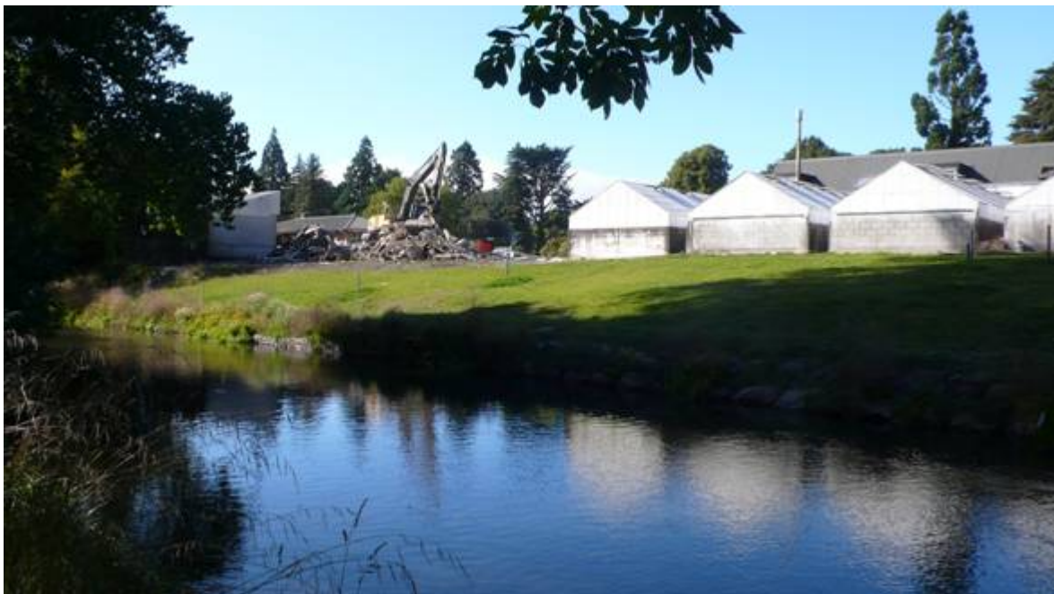
View across the Avon towards the site of the new Botanic Gardens Visitor Centre part way through demolition of the old nursery buildings.
