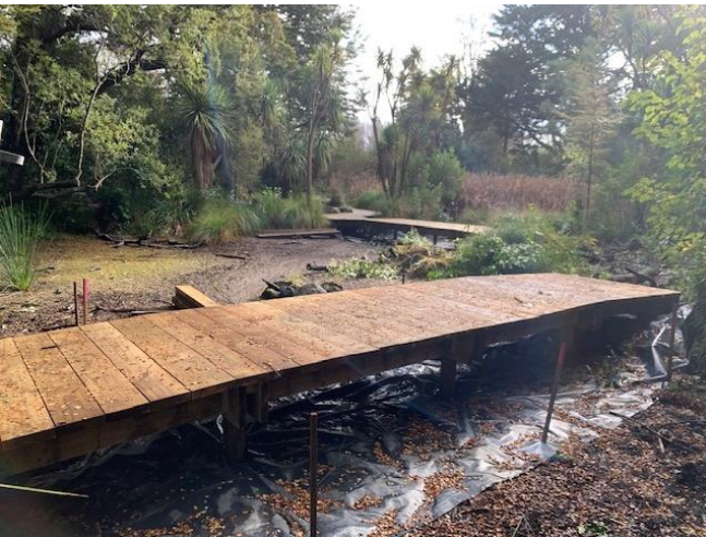
11: New board walk under construction between the Cockayne and NZ Icon Gardens.
