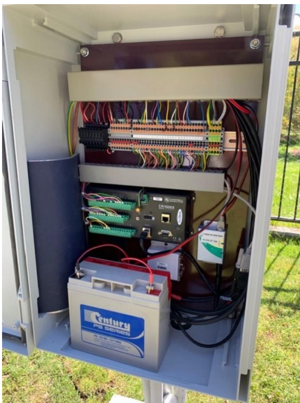
5: The new Weather Station Data-Logger
