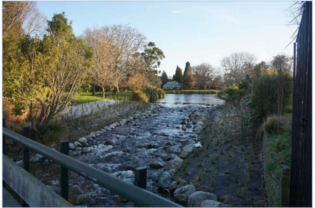
View of the newly completed water riffle, from the Latter Day Saints access bridge, the Mona Vale Homestead and the Bath House can be seen in the distance.
